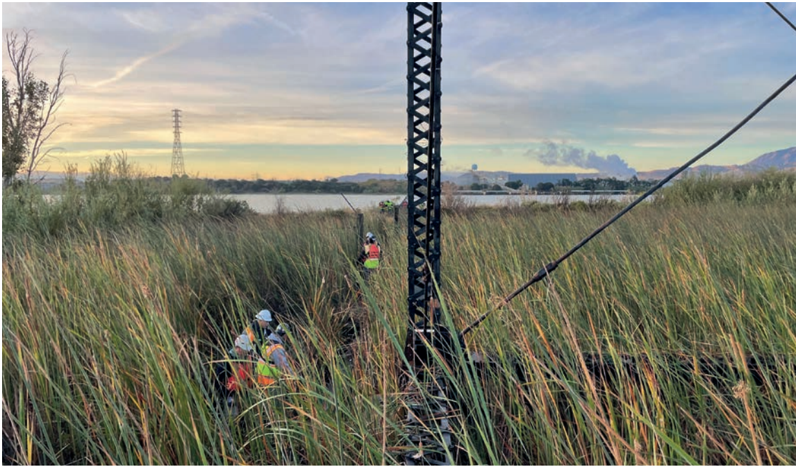
The demolition had to leave the surrounding marsh, wildlife and wetland intact and undamaged.
